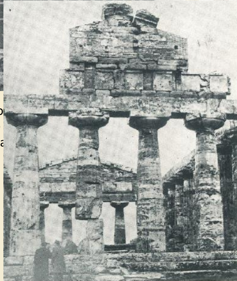
On the left: Few years after the intervention, during one rainstorm one thunderbolt hit the Temple, and one column exploded. The engineers (in the news paper picture on the left) were happy because their intervention, they said, saved the entire columnade.
