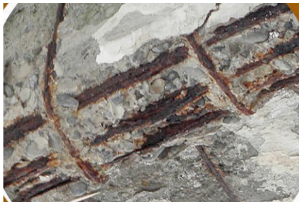
Fig. 4 – Barre longitudinali e staffe corrose in una trave in cemento armato - Corroded longitudinal bars and stirrups in reinforced concrete beam
